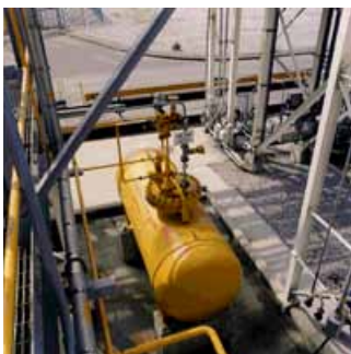
Expansion vessel mounted in a bund
