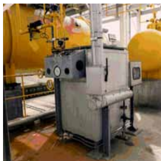
Coil in bath vaporiser heated by low pressure steam
