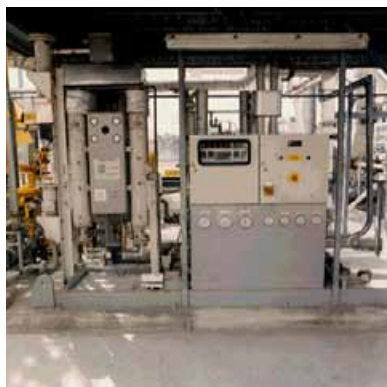
Air compressor unit
