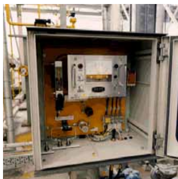
Hygrometer alarm. At this installation the compressed air dew point is less than -60^{\circ}\text{C}
